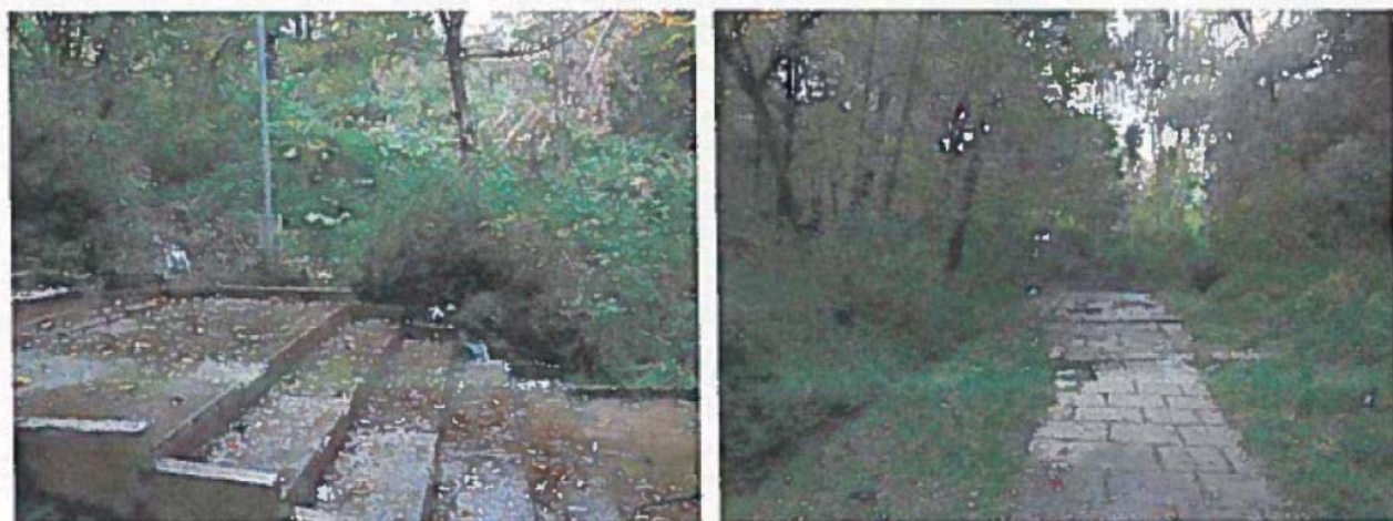
Fig. Aleea Paraul Sipote – Zone deteriorate
